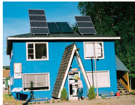
One Sky's office with 1.2 kW net-metered PV system and solar hot water heater.
